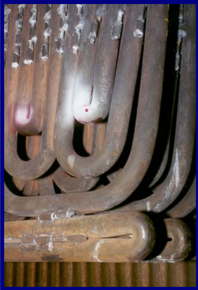
Superheater tube crack
